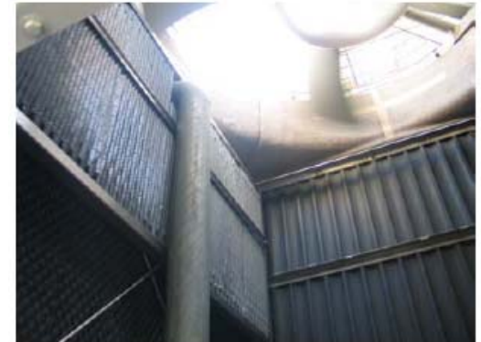
Drift eliminator not extended across whole air stream
