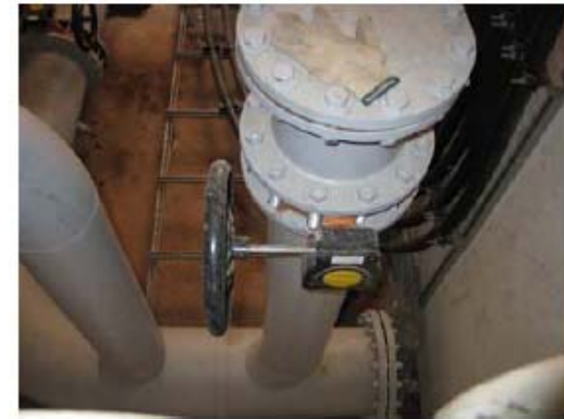
A long dead leg branches off from the main pipe
